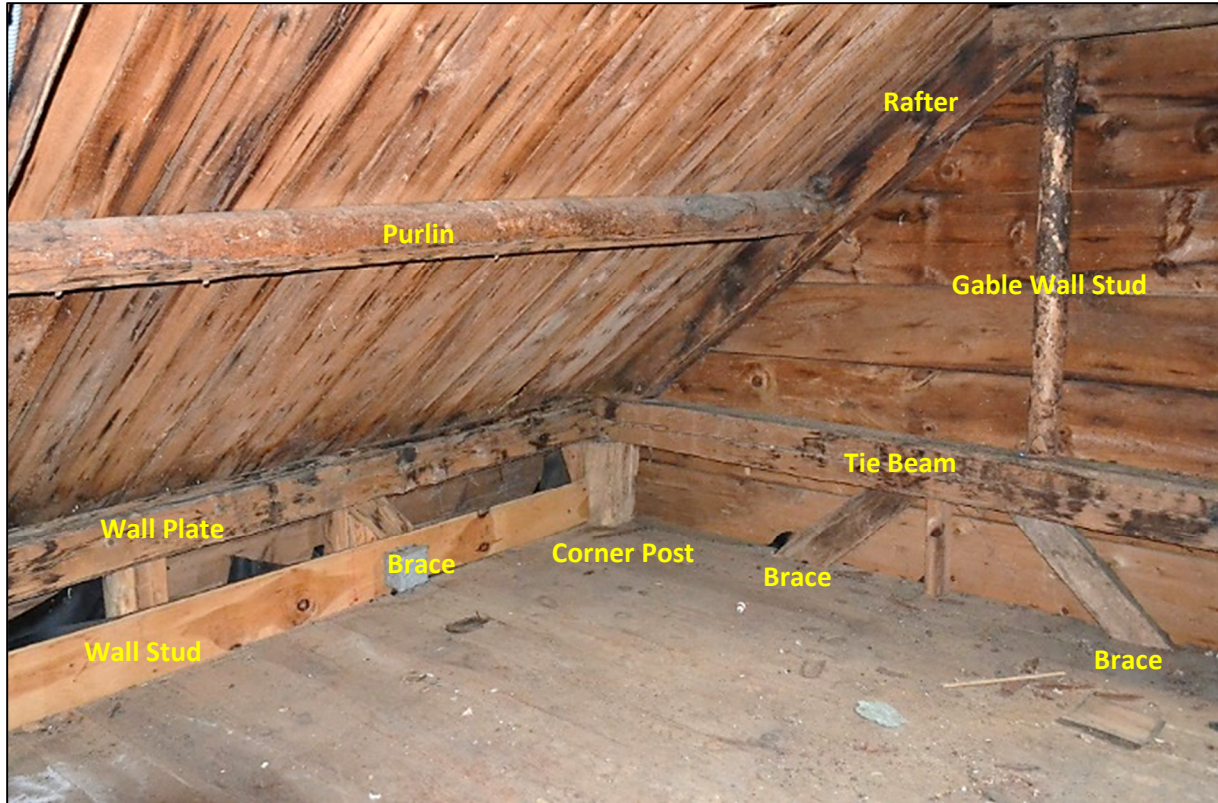
Northeast corner of shop attic, camera facing east. The framing of the kneewall is exposed.
