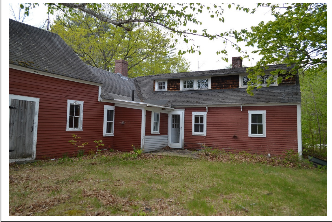
Photo # 4 Description: Rear frame (wing) attached to main house, showing added shed dormer Reference (file name or frame#): DSC0092 Direction: Camera facing northwest
